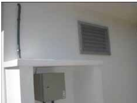
Ventilation opening to minimize the entry of pests.
