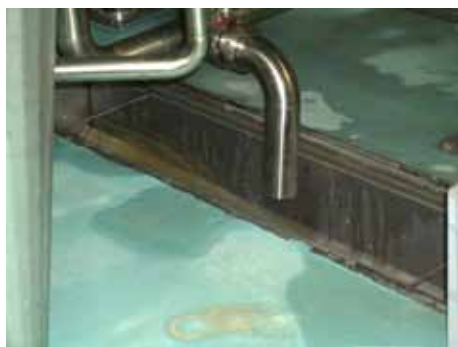
High capacity drain in a bottling area
