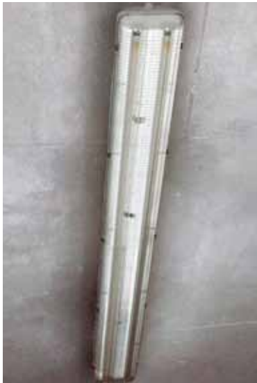
Artificial lighting with unbreakable cover
