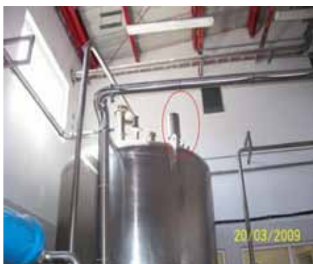
Water storage tank equipped with an air filter
